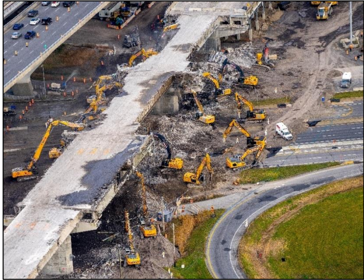
Demolition of spans above Hwy. 132 in 2022 which generated thousands of tonnes of materials
