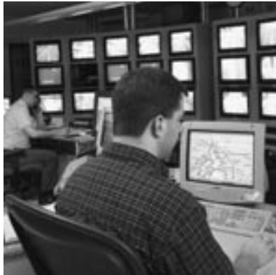
Video camera surveillance and lane signalling control room for the Jacques Cartier and Champlain bridges in Montréal
