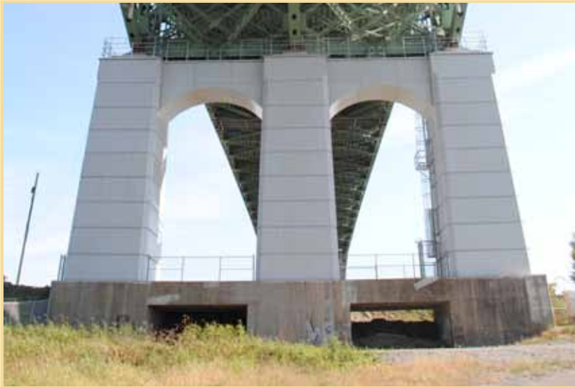
For the first time on the Champlain Bridge in Montreal, a steel form was used in the rehabilitation of one of the piers underneath the deck.
