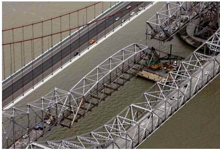
Figure 20 – Lowering of Suspended Span of the Carquinez Bridge (source: Courtesy of Foothills Bridge Co (Photo by Jakub Mosur))
