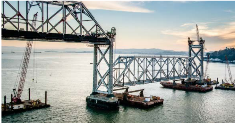
Figure 21 – San Francisco Oakland Bay Bridge – 504’ Span Dismantling Image Courtesy of Foothills Bridge Co (Photo by Sam Burbank)
