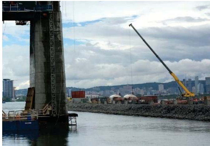
Figure 27 – View of the jetty for the construction of the new Champlain Bridge from the St. Lawrence Seaway dike (photograph taken on June 22, 2016)
