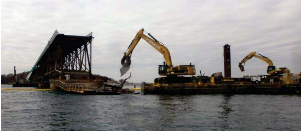
Figure 25 – Standard barge method used for the demolition of the Long Island Bridge in Boston Harbour (Source: Walsh Construction 2016)
