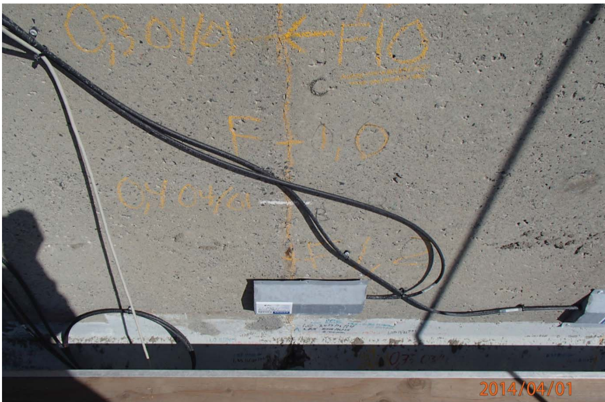
S5.PC.28W-29W.P7.n – 0490 (fissure F10 – centre face amont)
