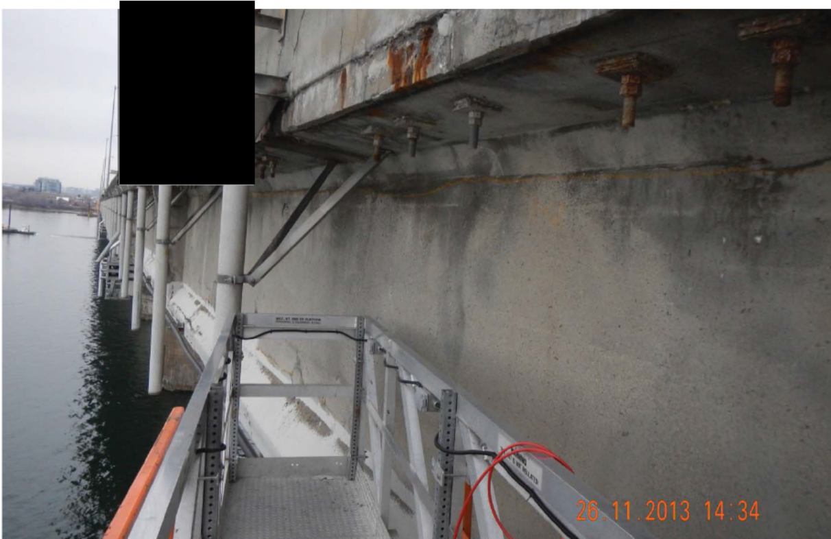
S5.PC.21W-20W.P7.c – 4367 (Fissure F5 - face amont)
