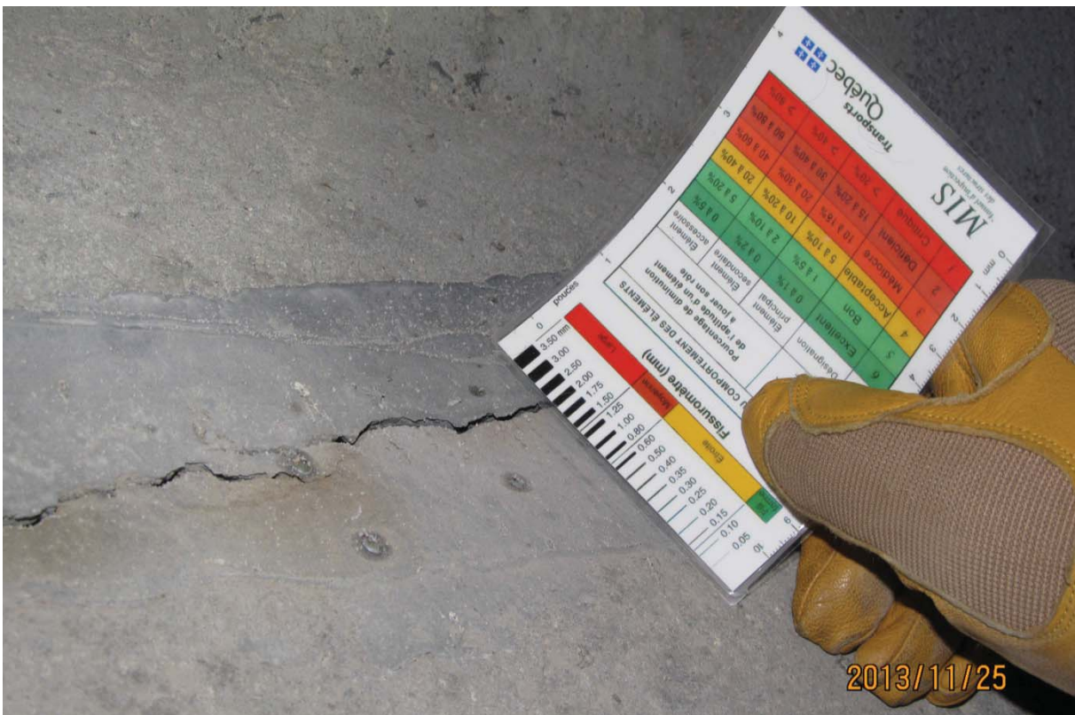
S5.PC.27W-28W.P7.f – 6418 (câble #24 – centre face aval)
