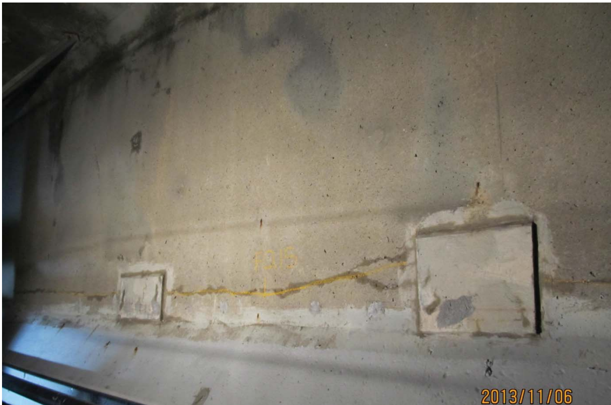
S5.PC.15W-16W.P7.d – 6152 (âme – centre face amont)
