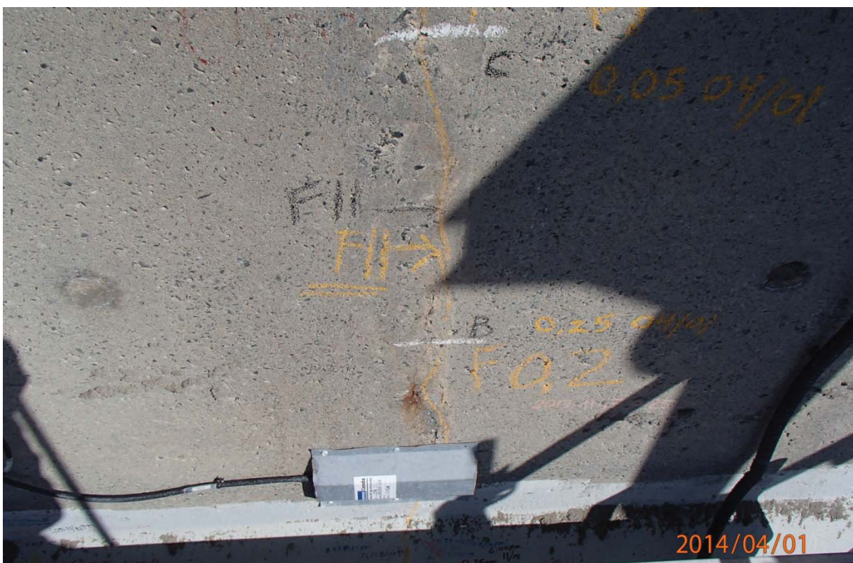
S5.PC.28W-29W.P7.o – 0485 (fissure F11 – centre face amont)
