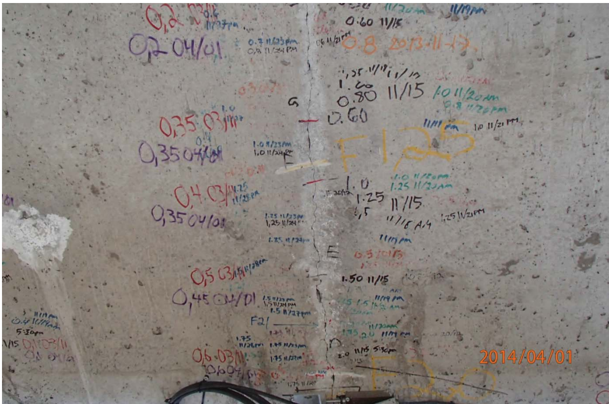
S5.PC.28W-29W.P7.r – 0478 (fissure F21 – centre face aval)
