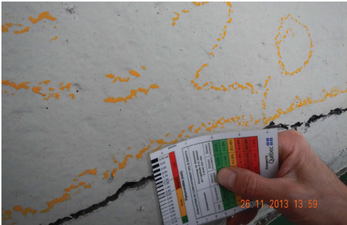
S5.PC.21W-20W.P7.e – 4356 (Fissure F3 – centre face amont)
