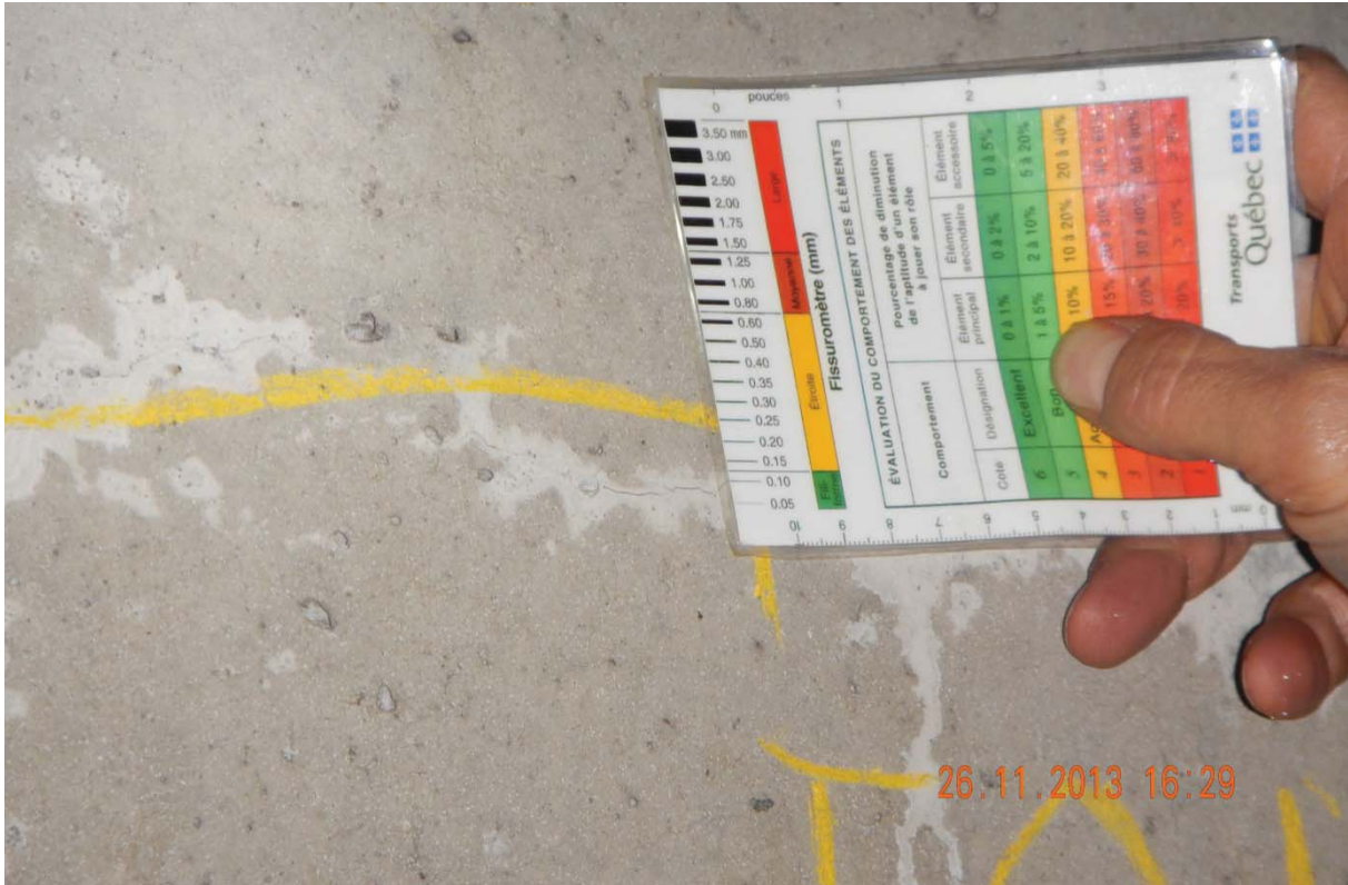
S5.PC.21W-20W.P7.g – 4390 (Fissure F9 – centre face aval)
