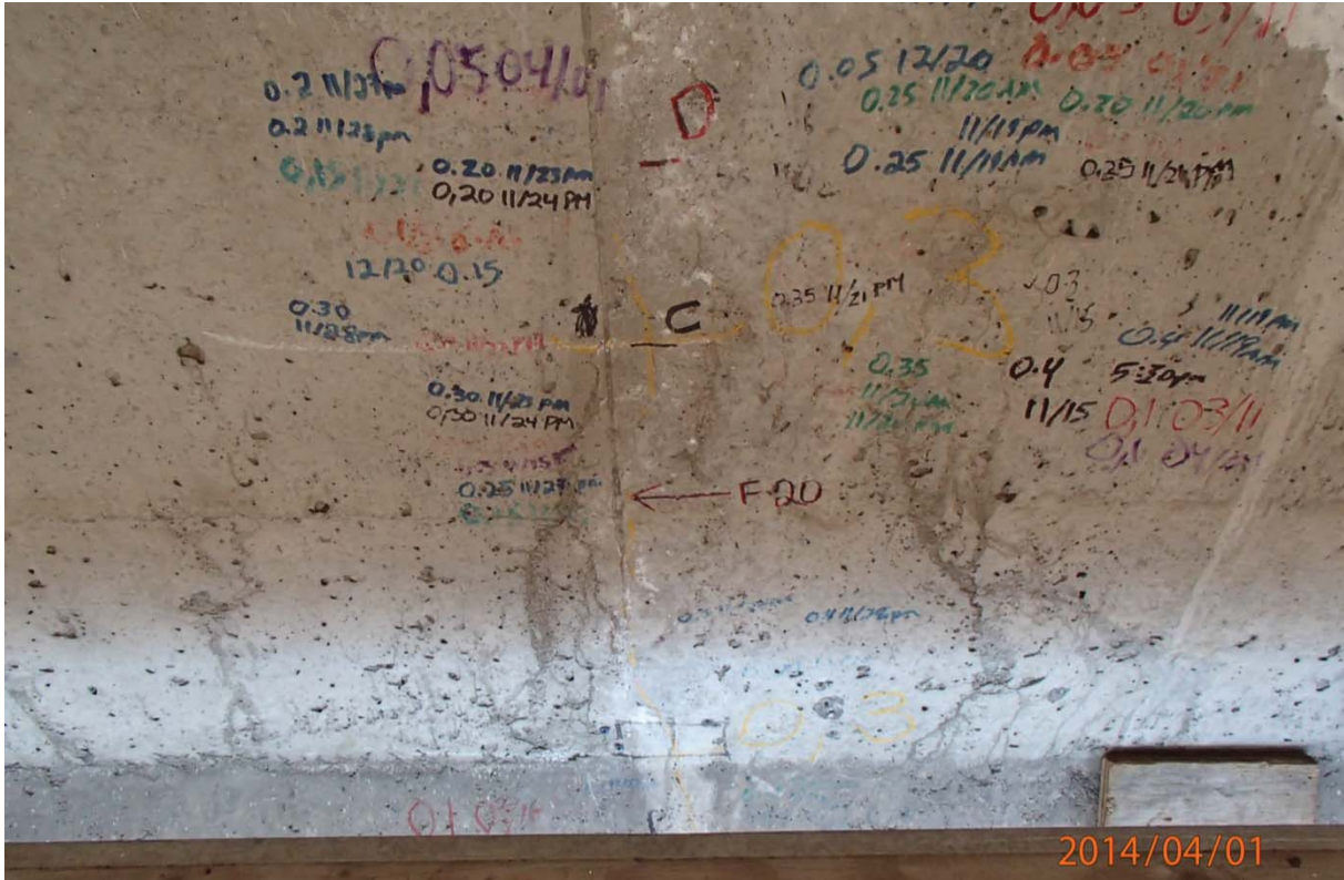
S5.PC.28W-29W.P7.p – 0474 (fissure F20 – centre face aval)
