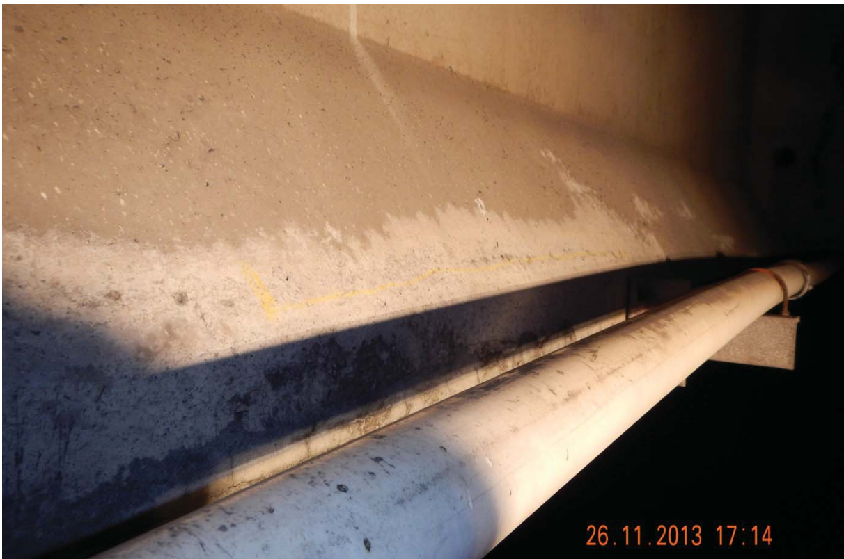
S5.PC.21W-20W.P7.h – 4395 (Fissure F10 – centre face aval)
