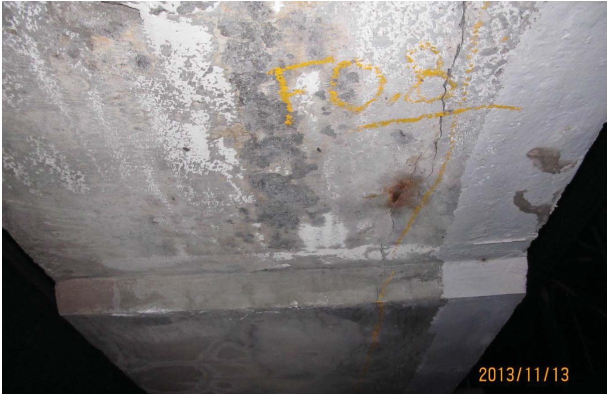
S5.PC.24W-25W.P7.e – 6274 (soffite – centre ouest)
