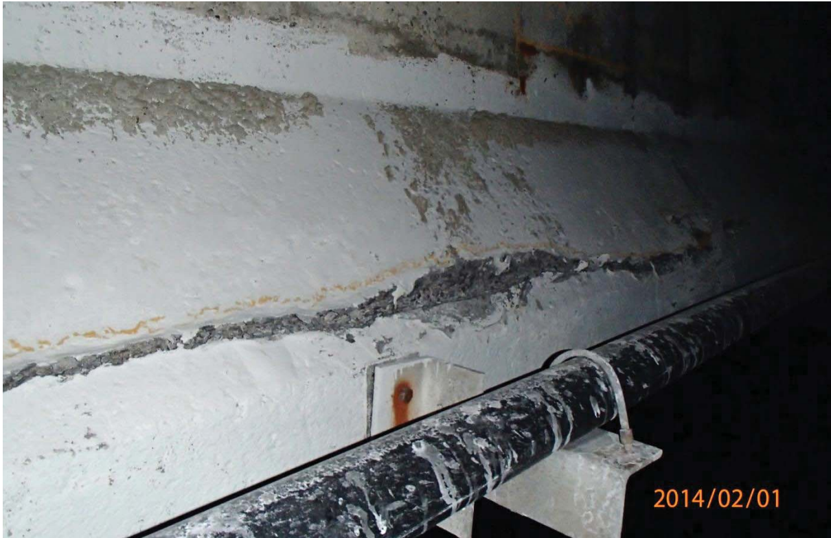
S5.PC.21W-20W.P7.a – 4359 (Fissure F4 - face amont)
