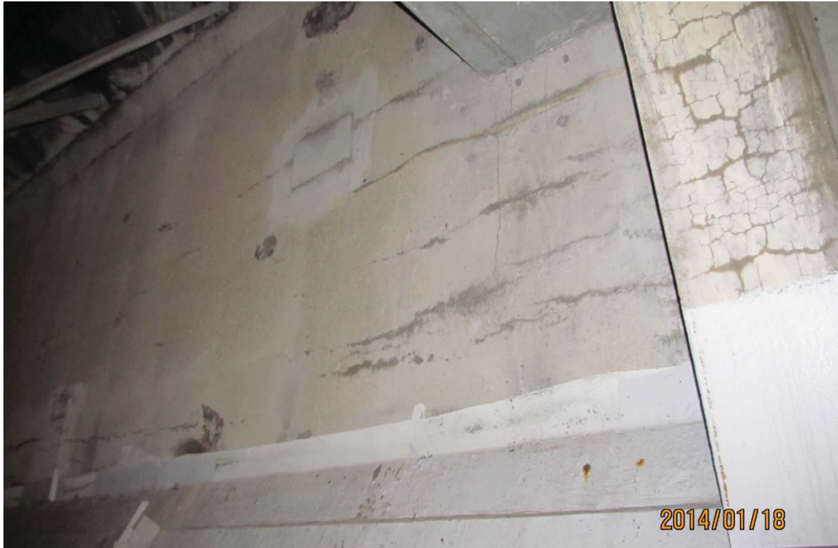
S7.PC.12E-13E.P1.c – 0183 (âme - centre ouest face aval)
