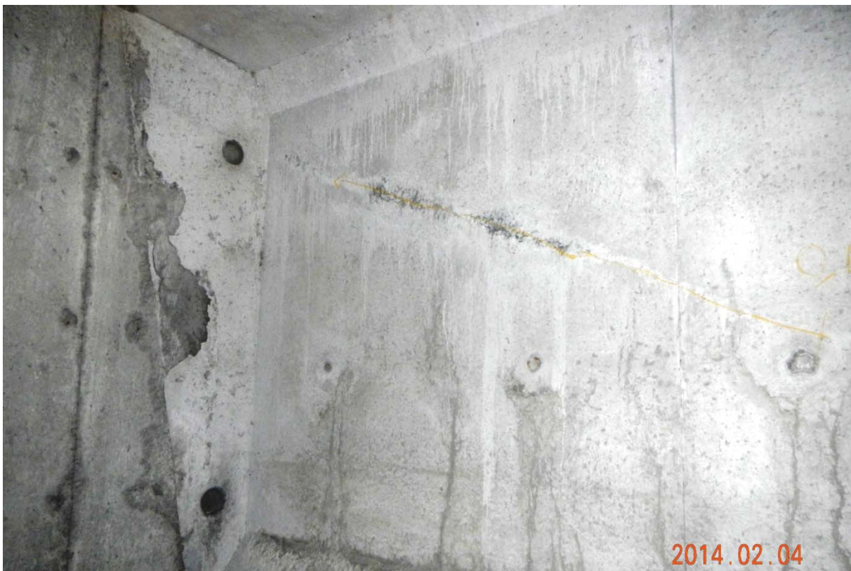
S5.PC.31W-32W.P4.d – 7501 (câble #24 – centre ouest face amont)
