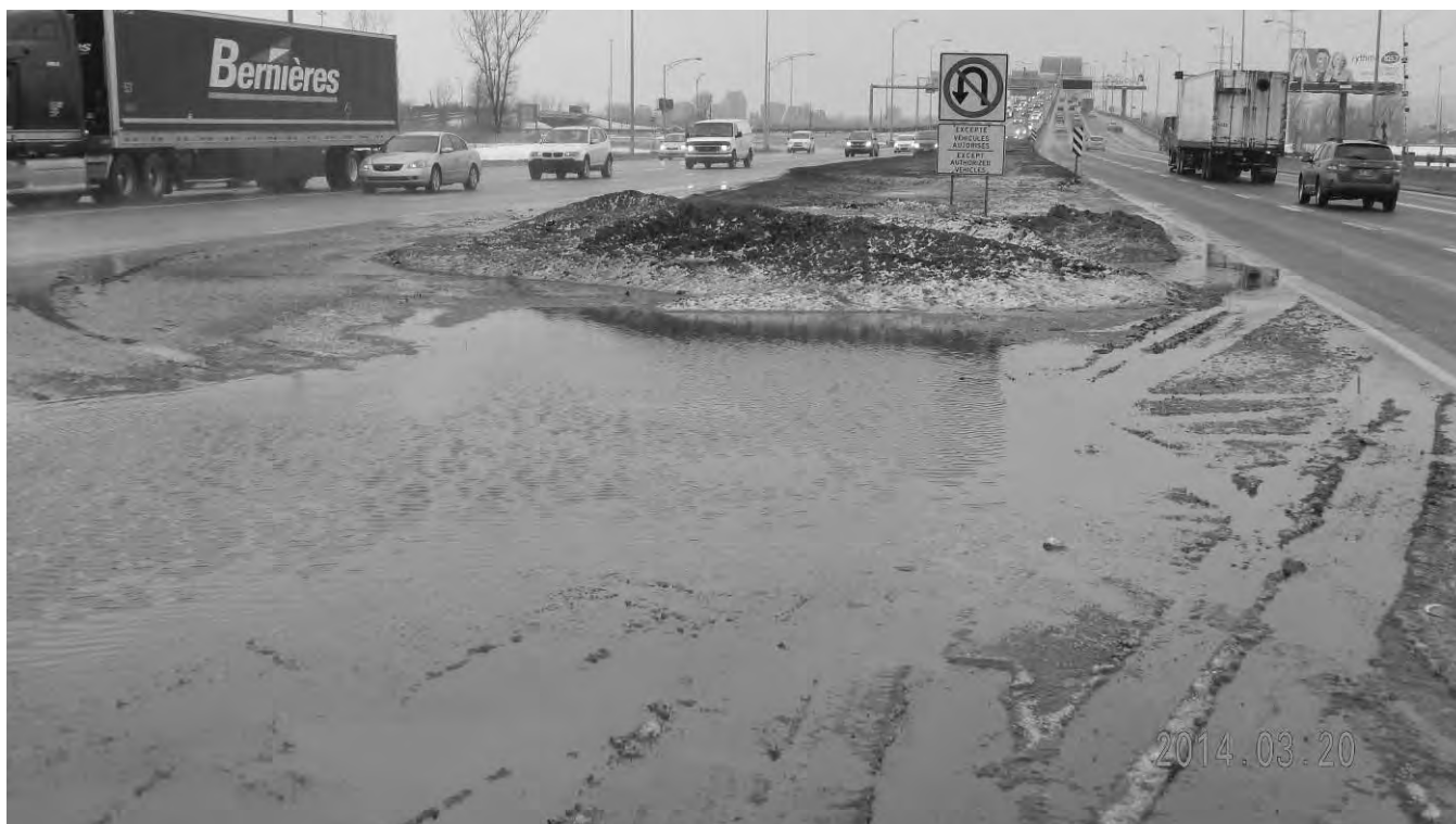
S8.Dr.4.a – 0313 – Drainage terre-plein
