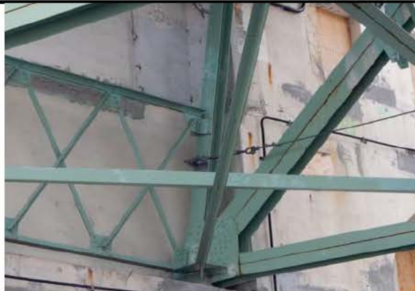
Photo 1: Montant L4-U4, face Nord JC_5_20160126_JM_8541
