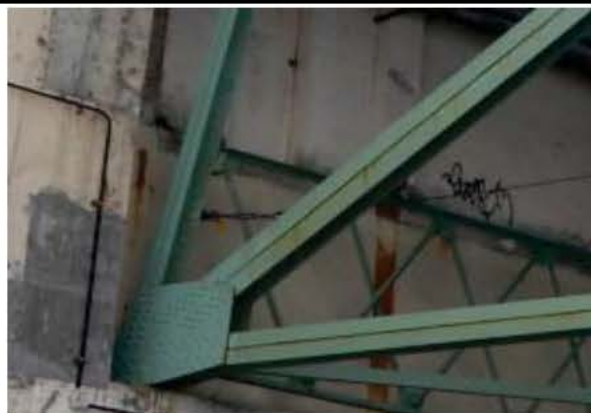
Photo 1: Montant L4-U4, face Nord JC_5_20160126_JM_8538
