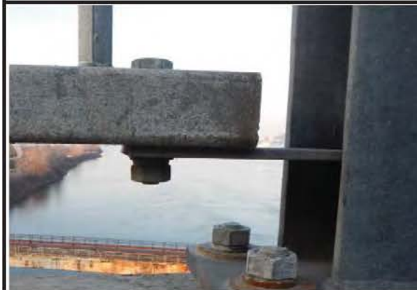
Photo 1: Dist. rive insuffisante JC_4_151125_JM_8238
