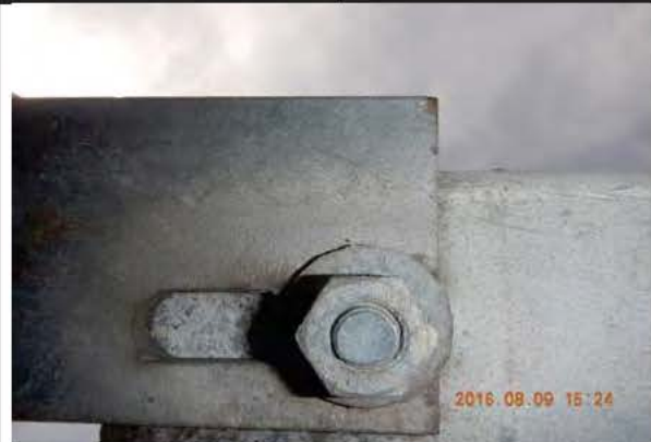
Photo 2: Dist. rive insuffisante JC_4_160809_JM_0047
