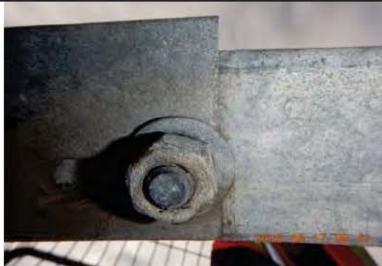
Photo 1: Dist. rive insuffisante JC_4_160817_7806
